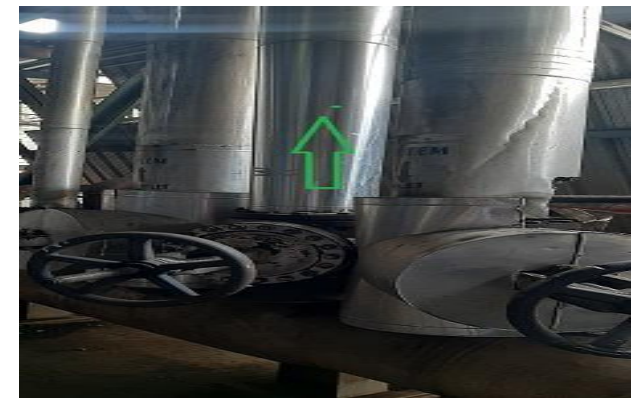
New Dedicated Dome Steam Line
